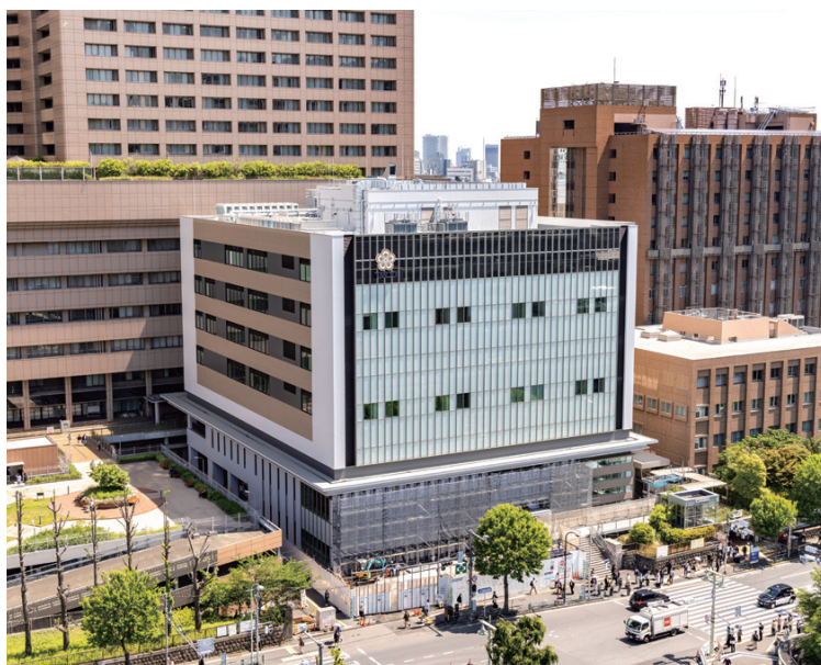
写真：工事中の機能強化棟 (地上7階、地下2階) Functional Enhancement Building under construction (7 floors aboveground and 2 underground floors)
